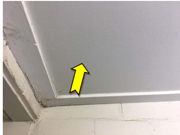
Photo 4. Interior, throughout, ceiling – suspected lead-containing white upper paint system.
